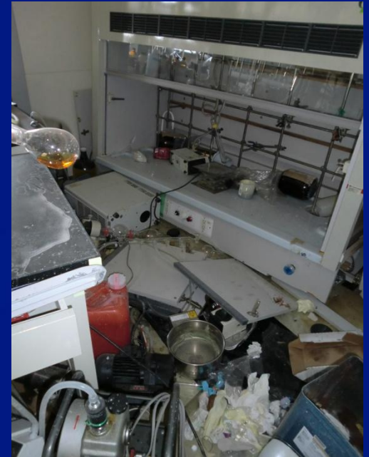
Japanese Earthquake: Fume hood was in fact torn from the wall
